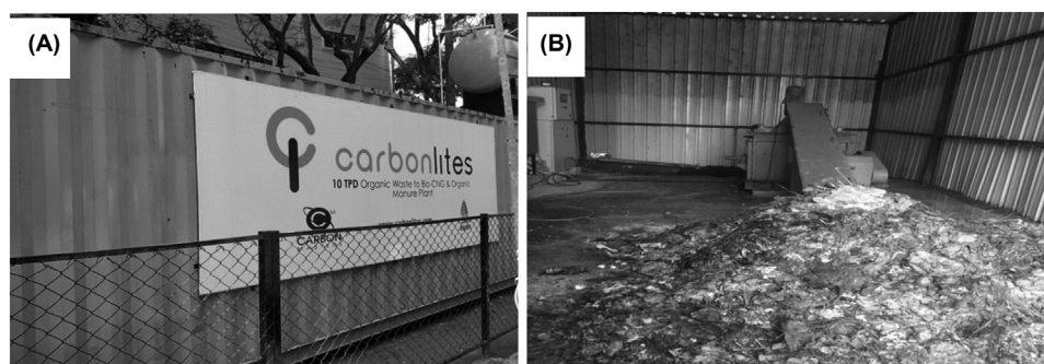
FIGURE 14.8 (A) Anaerobic Digester (refurbished 40 ft shipping container), (B) Shredder.
